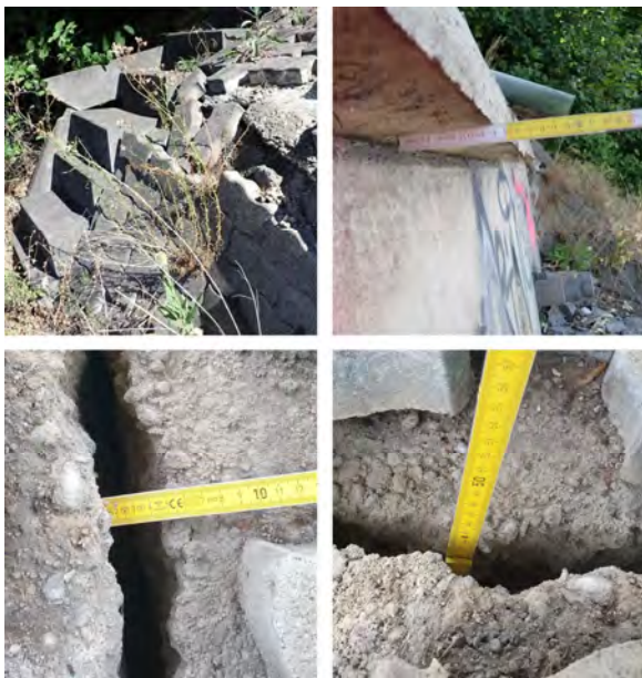
Figure 4. Deformation of the steps and crack measures.
